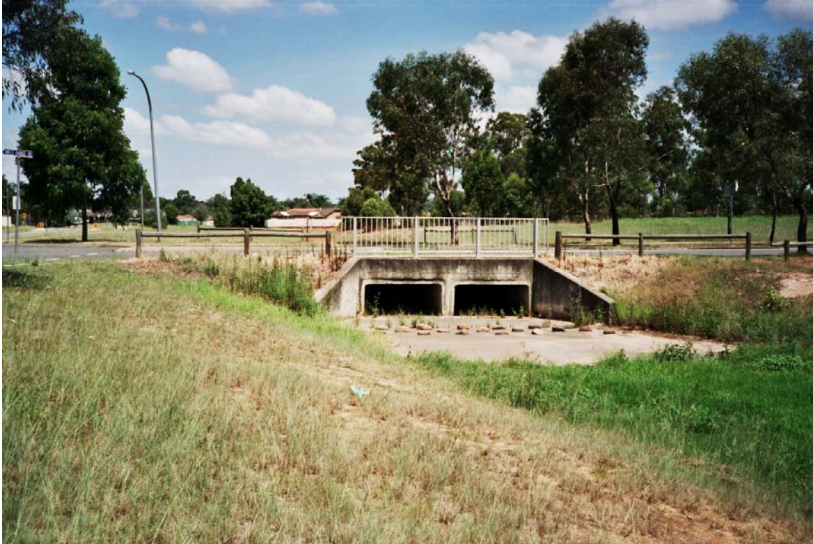
Photograph No. 2: View of BP12 and Rifle Range Road twin box culvert structure, looking upstream.
